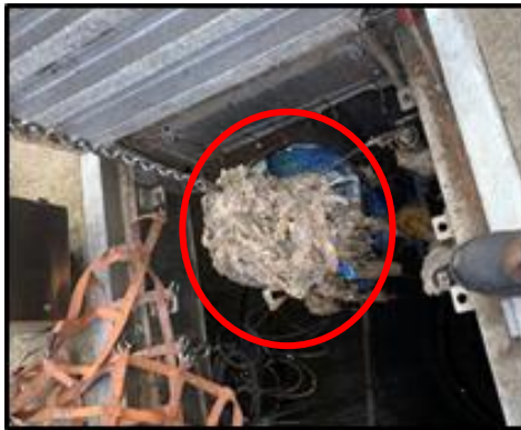
Accumulation of rags onto of submersible pump.
