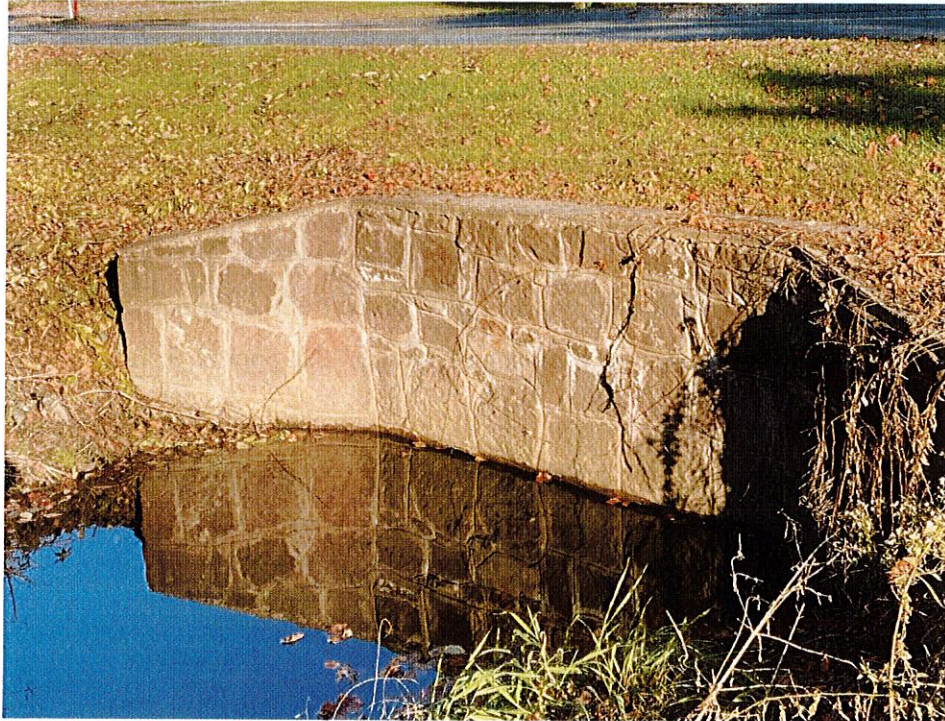
Figure 8: Newberry Brook culvert under Main St looking north, 11/8/2021. The two drainage pipes are completely beneath the water level on the downstream side.
