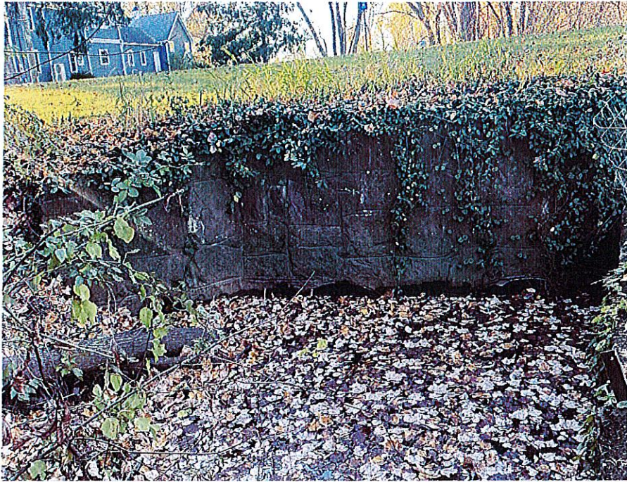
Figure 7: Newberry Brook culvert under Main St looking south, 11/8/2021. The tops of the two drainage pipes are just visible above the water level on the upstream side.
