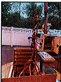
On-call operators responded to an alarm at Avery Street Pump Station to find a pump had detached from the guide rails resulting in pump damage, inoperable level floats and tangled cords.
