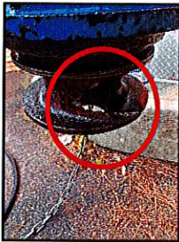
Damage to the Avery Street pump impeller. The maintenance staff replaced the impeller and volute before putting the pump back in service.
