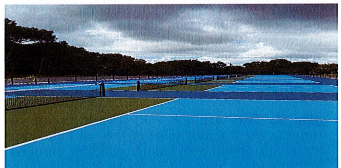
Getting close to opening. Waiting on some, fencing & Parks crew will add parking and ADA accessible areas along with heavy-duty wood guardrails.
