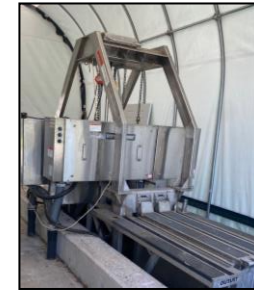
Existing UV Bank that has been in service for 20 years.
